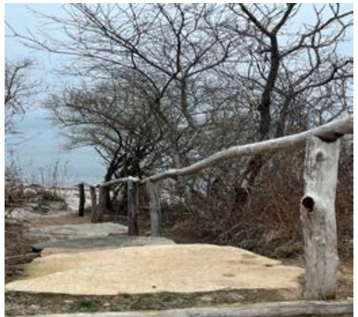
New railing constructed by F.I. School students with stone steps installed by Race Rock Co. Photo by Jack Schneider.
